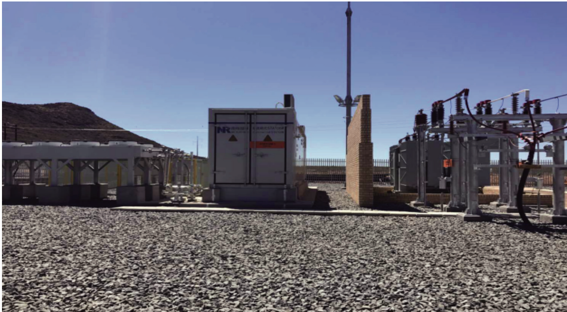
STATCOM picture on site
